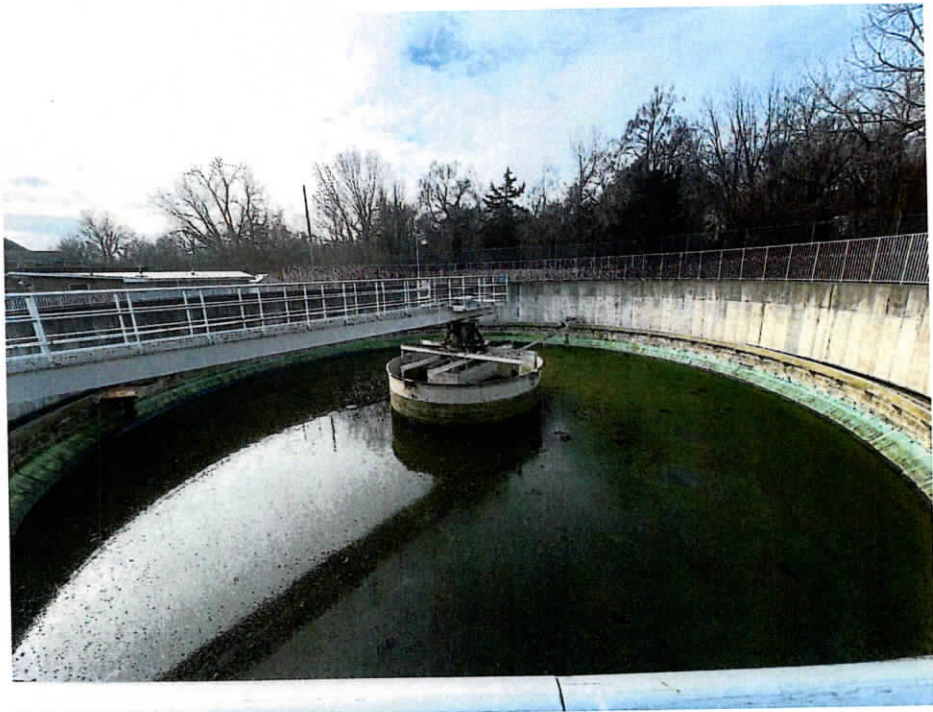
Figure 4 Inoperable Secondary Clarifier
