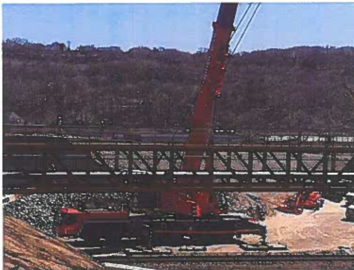
Figure 16 Ansonia Riverwalk Park, pedestrian bridge construction April 2018, Photo by Michael P. Mayko CTPOST
